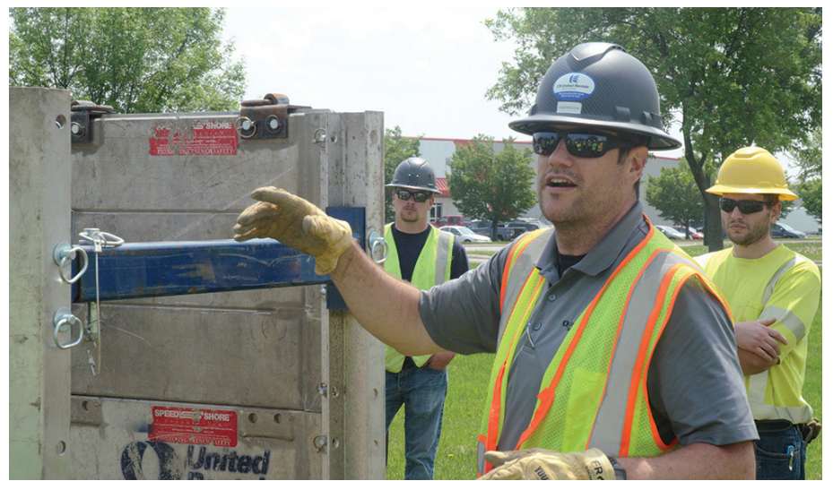
Joel DePons talks about the correct way to assemble a trench box.
