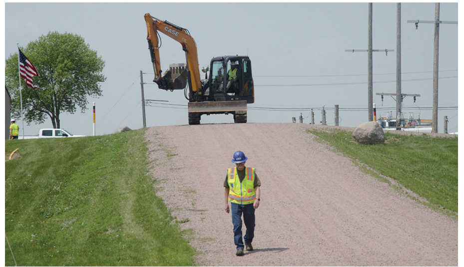
Andy Smoka led the excavator, driven by Tommie Flores, down to the training field.
