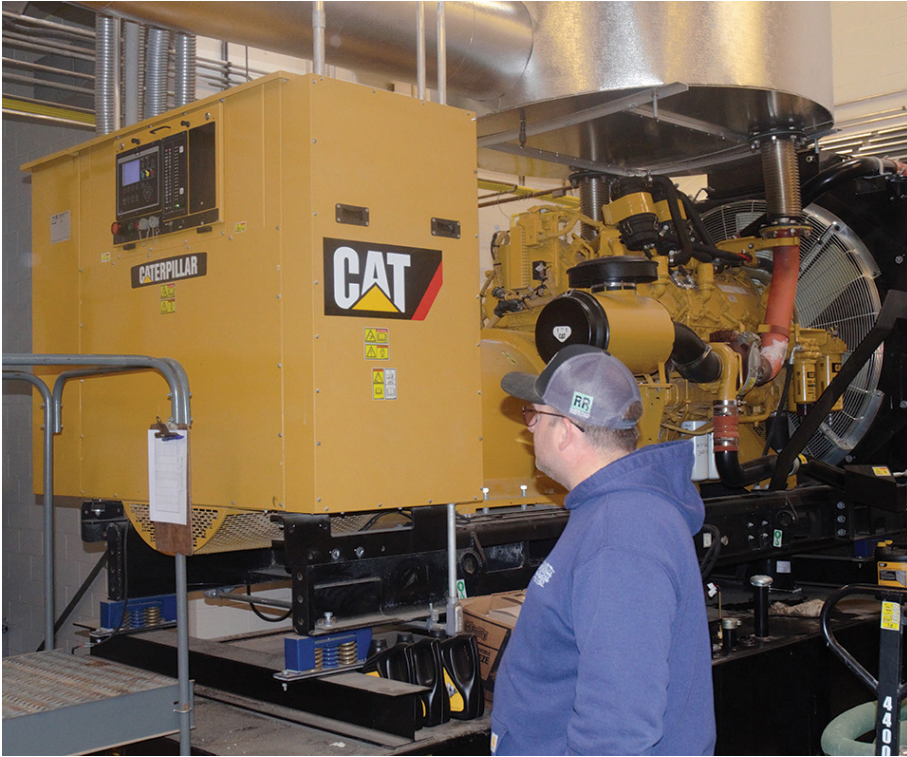
Tim Anderson of Marshall Municipal Utilities examines the 800-kilowatt Caterpillar backup generator for the water plant.
