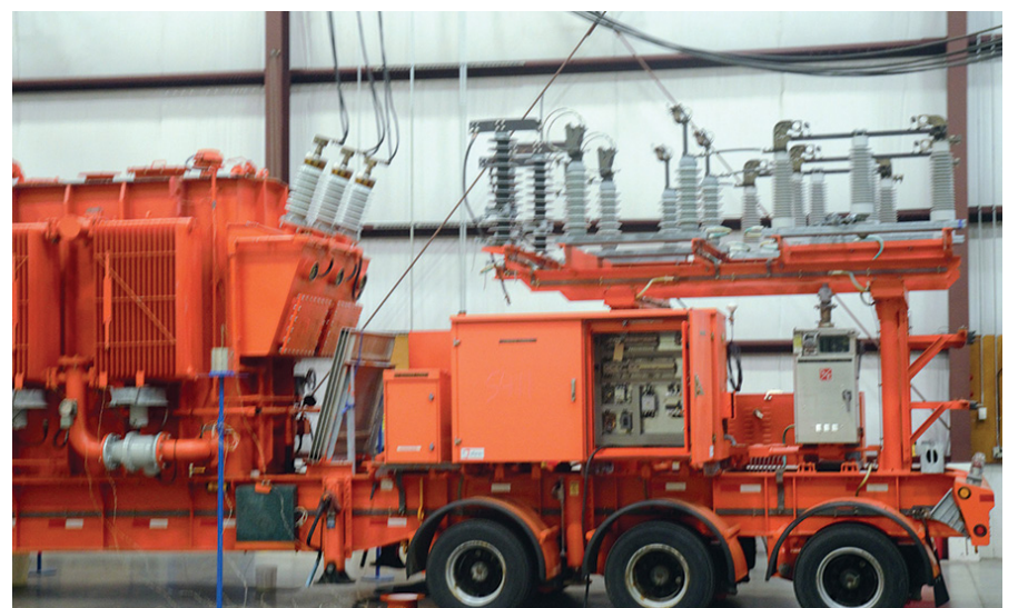
A Portuguese-built mobile substation gets an overhaul at Jordan Transformer.
