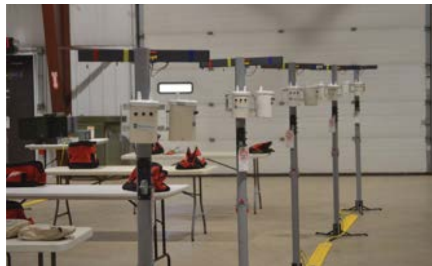
The miniature transformer banks are an excellent tool for learning about transformer connections.
