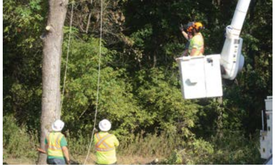
Jay Reading, MMUA's assistant director of Technical Services, and a learner size up a cut before going up in the bucket.
