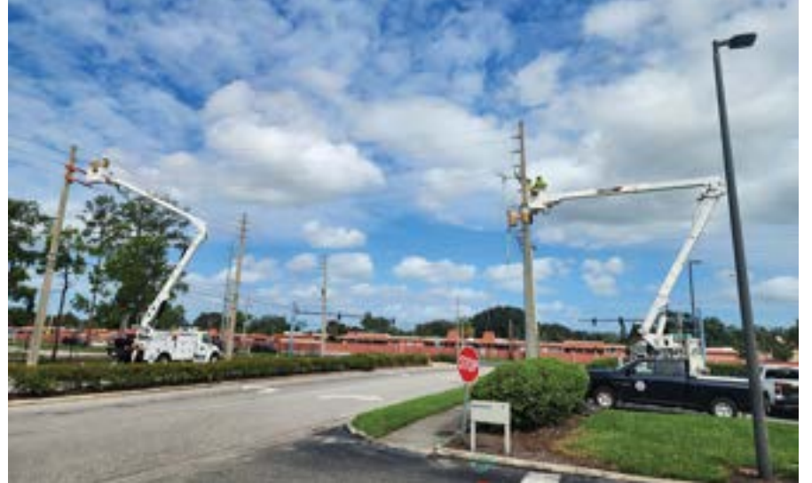
The crews restringing phases across the road and rebuilt a transformer bank.
