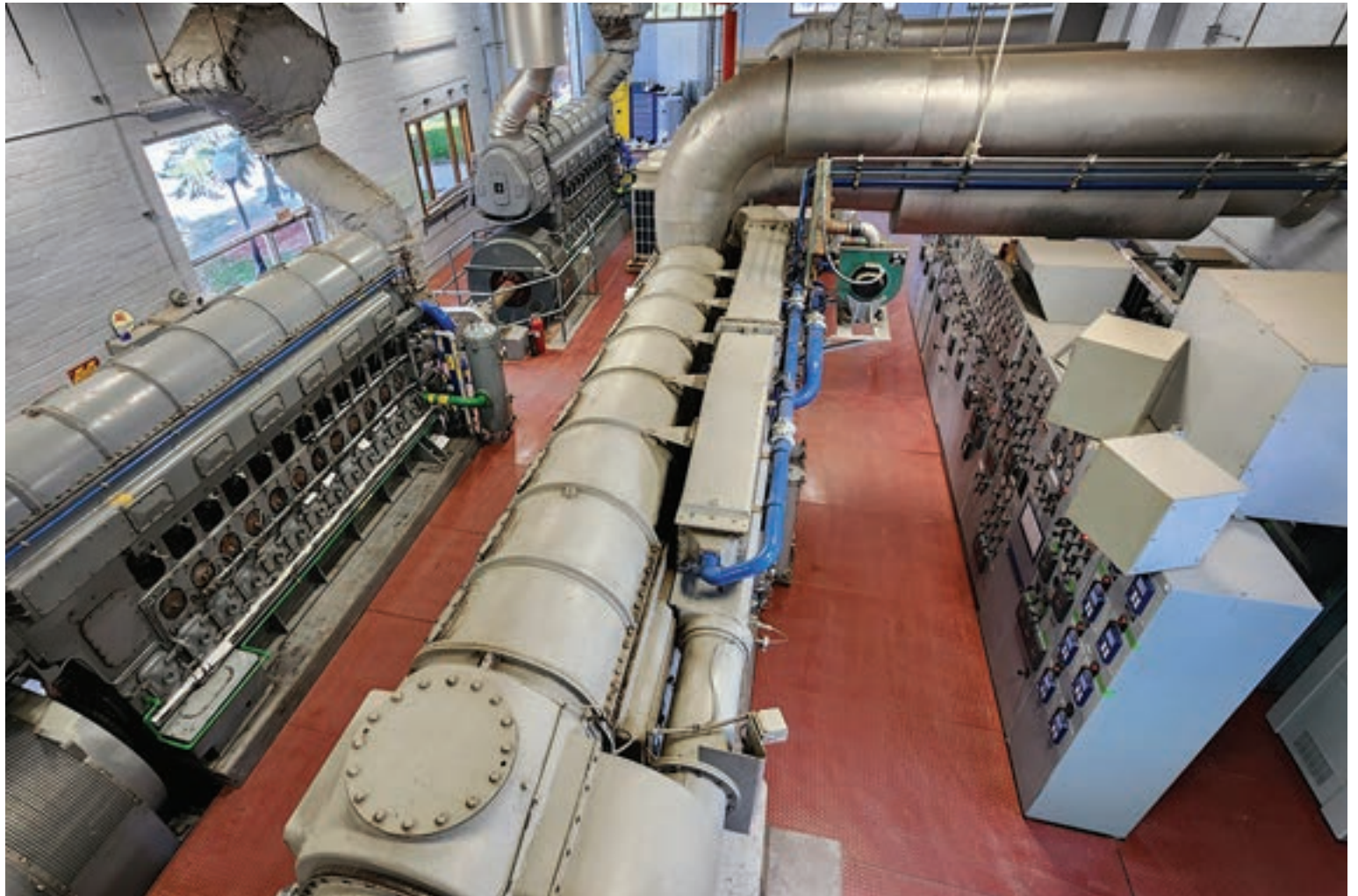
Delano’s power plant got a workout on the evening of August 26, when a prepared DMU kept the lights on for the City of Delano and several neighboring communities.
