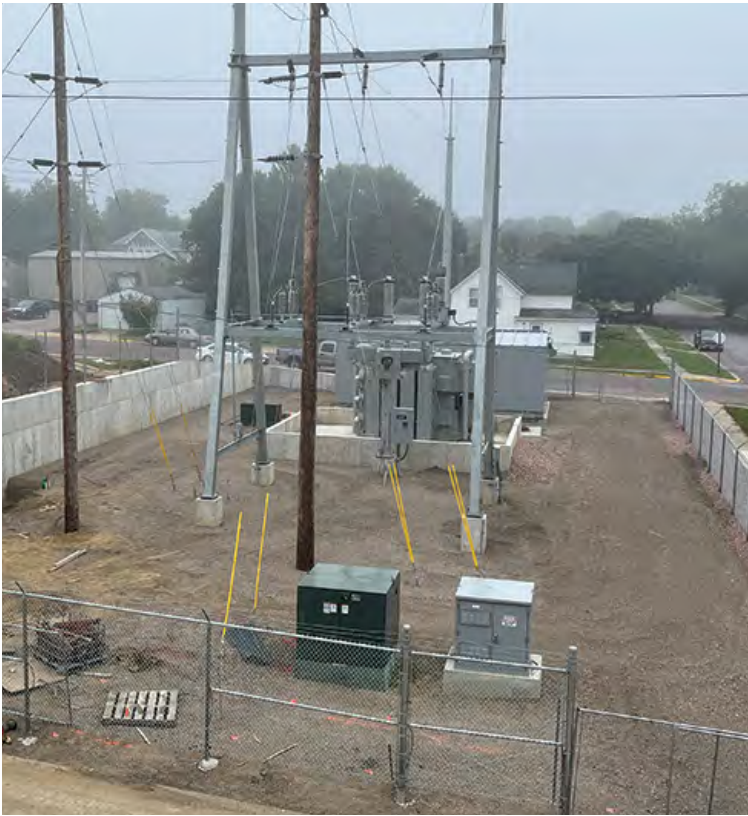
The most recent image of the new substation site is from August 2024. It shows significant progress. Transmission poles have been installed. The north wall has been completed. At this point, the project is nearly ready to energize but is currently on hold due to pending safety checks, primarily because the fencing needs to be completed.
