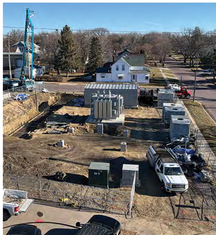
This photo, from December 2023, captures several details: Manholes are positioned to the right, ready for placement. Footings are being poured for the north wall. A-frame foundations have been set in place. A recently installed PMH 9 switch sits near the fence next to a metering enclosure.
