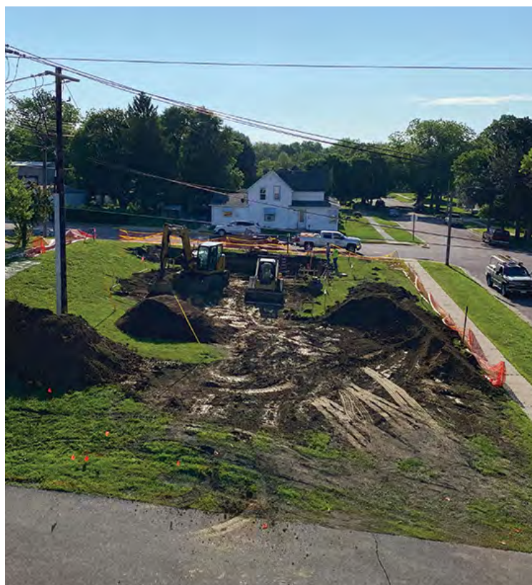
This photo series shows the completion of Madelia's new substation. In the first photo, taken in June 2023, the initial excavations are shown. At this stage, Madelia was preparing for the delivery of the 15/28 MVA transformer, which was expected in two weeks.
