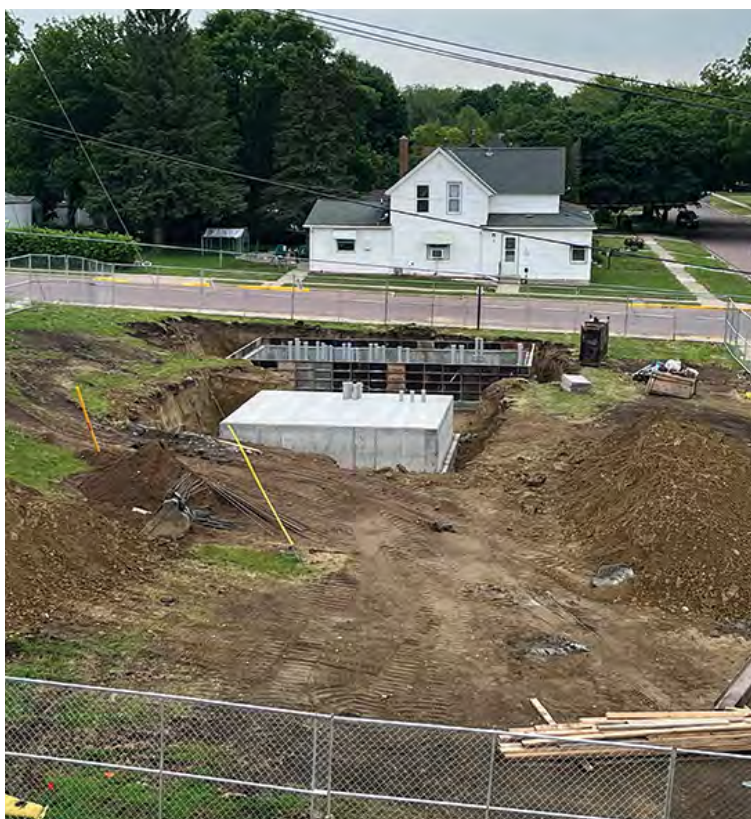
In this image, from June 2023, the pad where the new transformer would be placed has been poured. The forms behind the pad are for the switchgear building, scheduled to arrive in July 2023.
