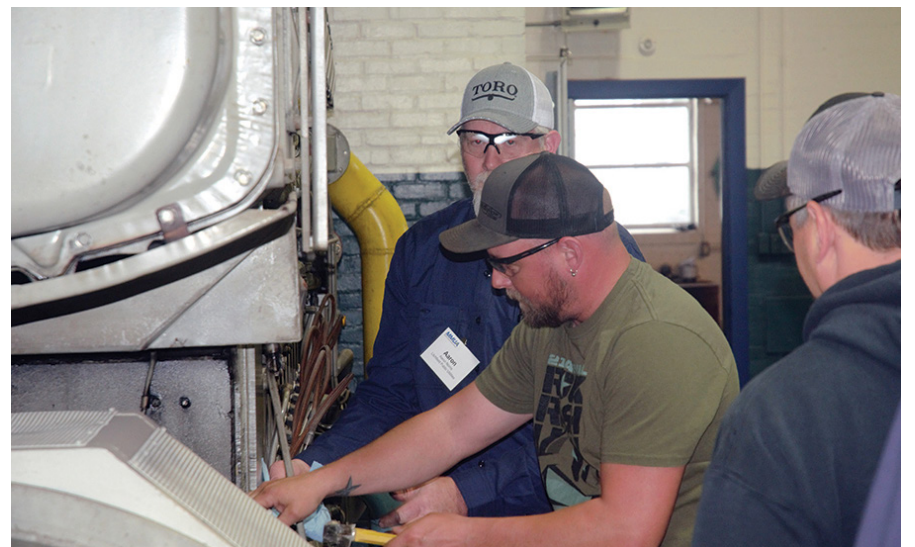
At the downtown power plant in Blooming Prairie, attendees focused on Fairbanks Morse generation.
