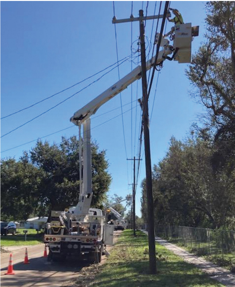
Tyler works in a bucket truck restoring power after Hurricane Ian struck Florida in 2022.
