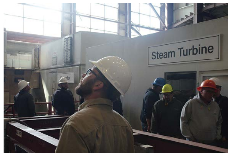
Attendees check out the steam turbine and the generator in the main building.
