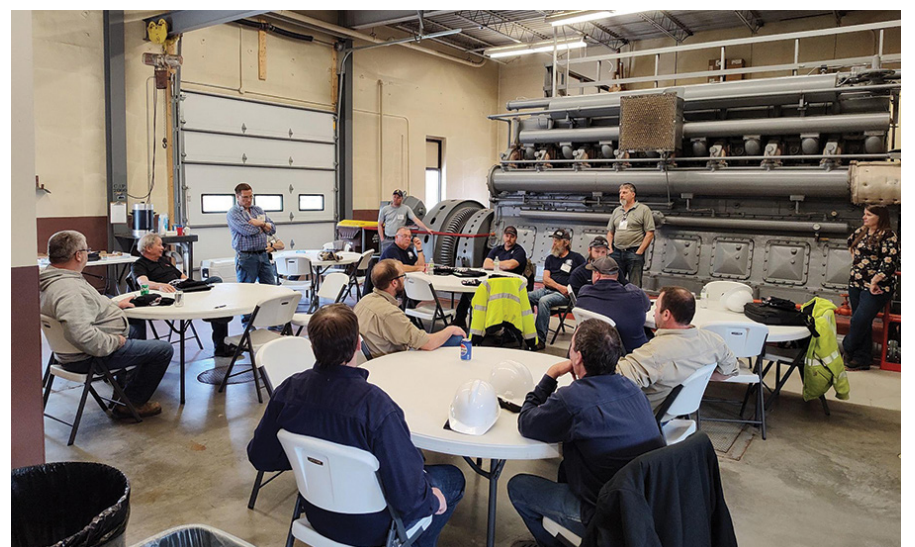
At New Prague Municipal Utilities, attendees discussed Cooper generation.
