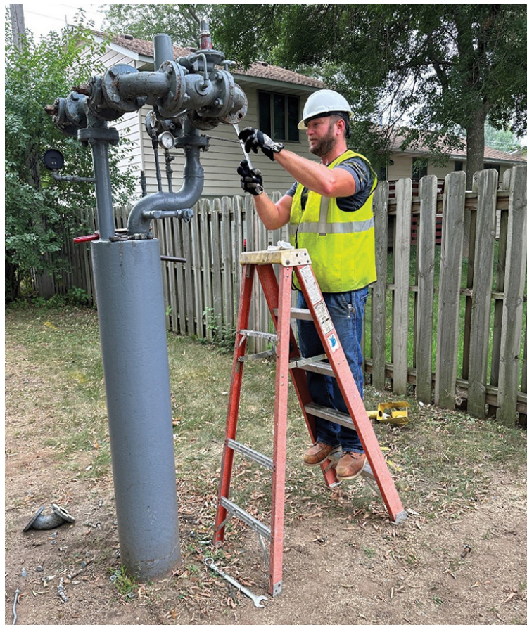
An Austin Utilities Gas Service Technician completing routine maintenance on a district regulating station (DRS). (Photo courtesy of Austin Utilities.)
