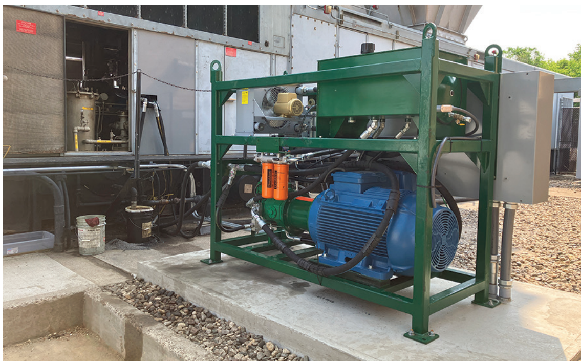
The new "skid", the electric pump and starting motor that replaced the 1968 Cummins Diesel.
