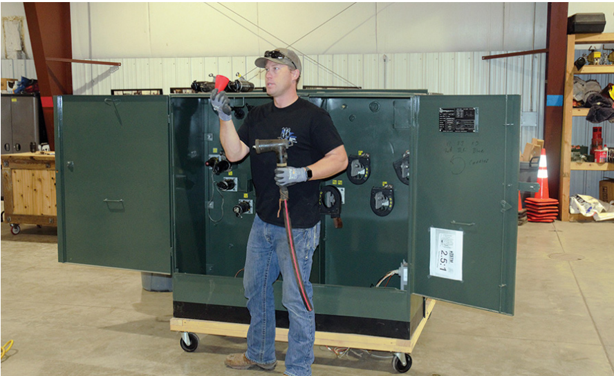
Cody shows learners the inner working of an electrical enclosure.
