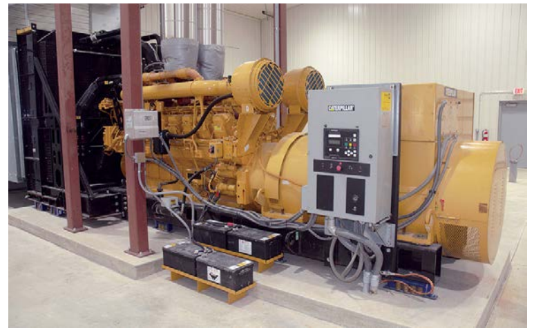
Blooming Prairie's newest generator came online in the fall of 2022. The #7 is a Caterpillar producing 1.8 MW.
