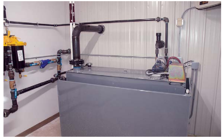
The day tank holds fuel pumped from the large outside tank to service the #7 generator at the Blooming Prairie Industrial Power Plant. It holds 235 gallons and is designed to warm the diesel fuel to keep it from gelling.
