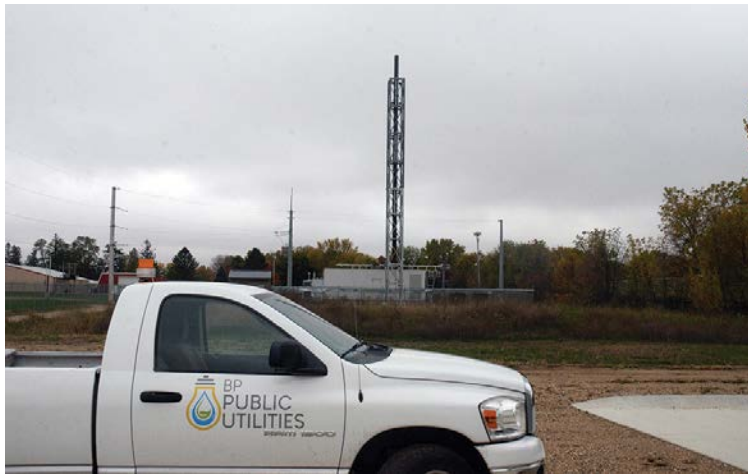
Blooming Prairie's #6 generator is a Cat-in-a-Box placed onsite at the industrial park.
