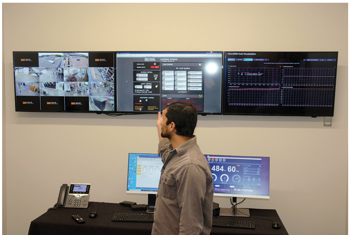
An employee shows attendees the Center's control room.
