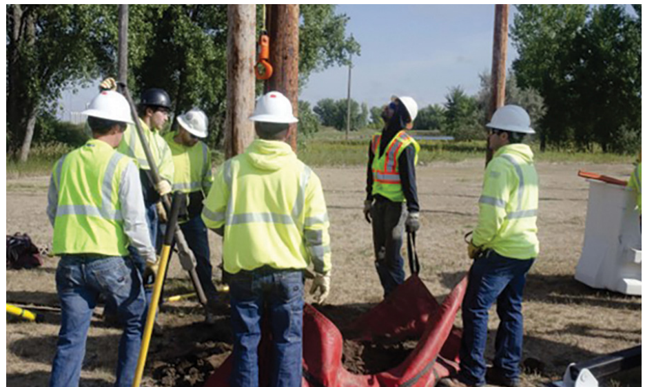
Students work to change out a power pole at the backyard easements and construction station.
