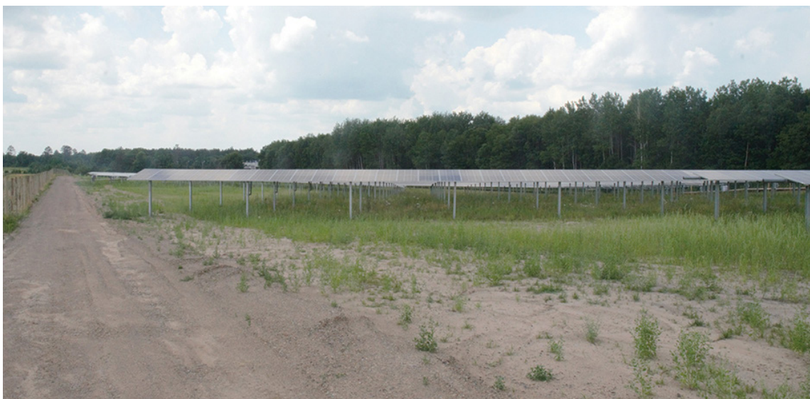
Brainerd's solar arrays consist of almost 14,000 solar panels.
