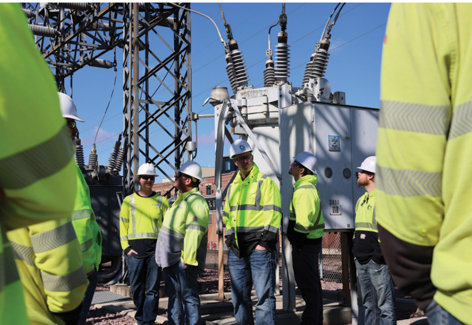
Through a combination of classroom instruction and guided substation walkthroughs, MMUA's Substation School helps utility professionals build the knowledge and skills needed to safely operate and maintain electrical substations. Classroom concepts were reinforced through hands-on, real-world application.
