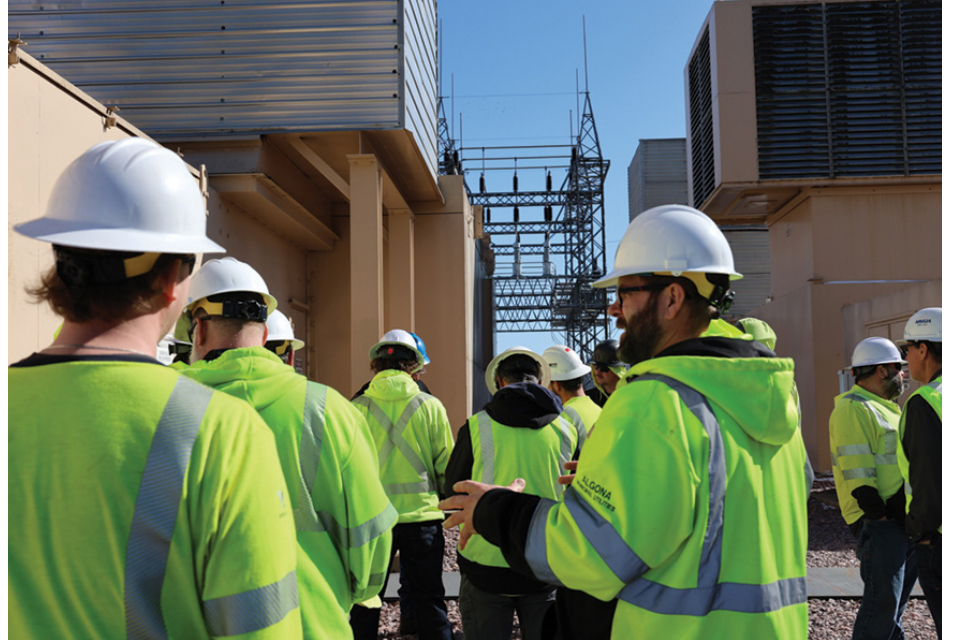
The next stop on the tour was the New Ulm Substation, located near the power plant. Participants toured the active substation, observing equipment layouts and discussing safety practices in a guided, controlled field setting.
