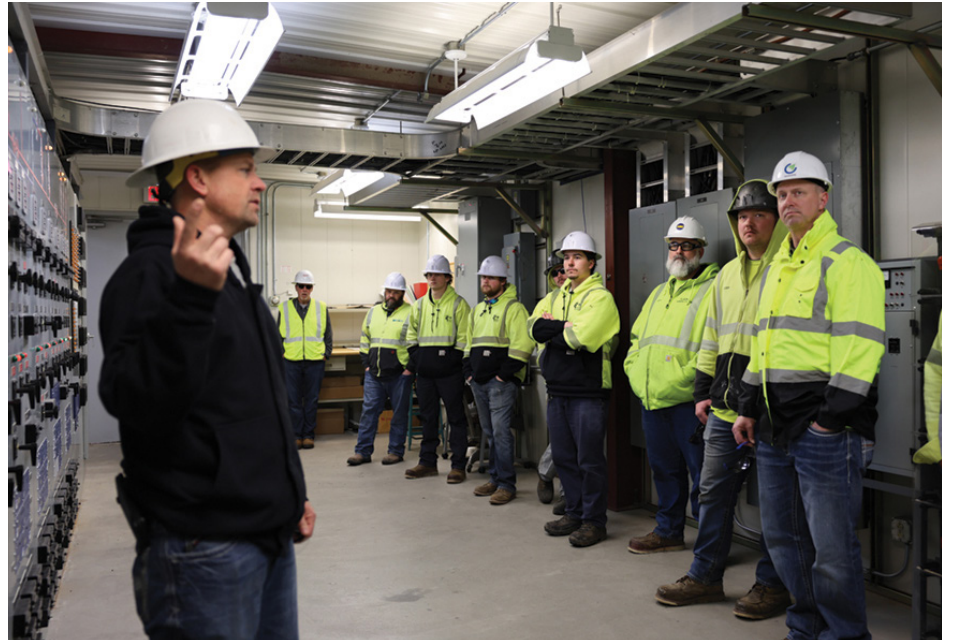
New Ulm Public Utilities' Gary Beranek leads participants through the substation control room, examining equipment and system functions while reinforcing hands-on learning through discussion and observation.
