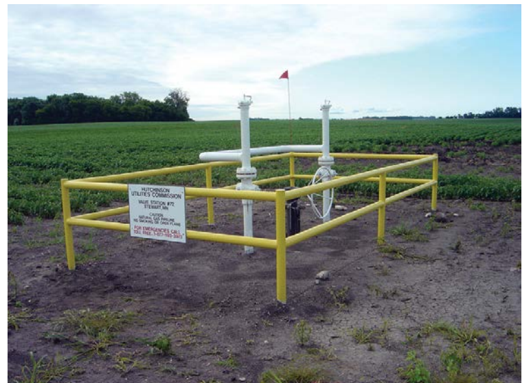
Natural gas distribution lines like these are under the greatest strain during prolonged cold snaps, when volatile fuel prices force utilities to decide whether to draw down reserves or pass higher costs on to customers.
