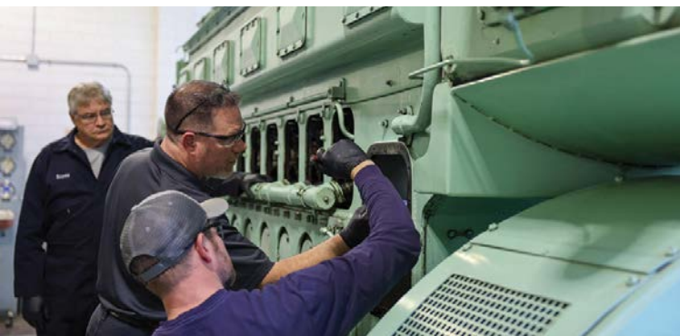
Brian King, Senior Training Instructor at Fairbanks Morse Defense, stands in front of Madelia Light and Power's Fairbanks Morse Engine while explaining the inner workings of a generation unit to attendees of MMUA's Generation School. Attendees of the school engaged in hands-on learning at three locations, each offering a different engine type. These included Cooper/Enterprise at SMMMPA's Fairmont Energy Station, Fairbanks Morse at the Madelia Power Plant, and Caterpillar at the Saint James Power Plant.
