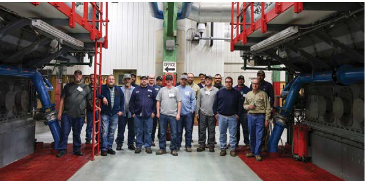
At SMMMPA's Fairmont Energy Station, one part of the split group stands for a photo between the two Copper natural gas generators. Bob Heine, a retired SMMMPA employee, led the training. As a former plant worker, he offered insights into the engines and inner workings of the energy plant.
