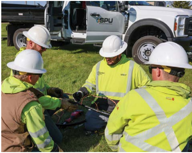
During the 200-amp terminations session, participants practiced terminating underground wire and learned to select the right tools for the job. Instructors covered skirted terminations for risers, 200-amp elbows, and splices.
