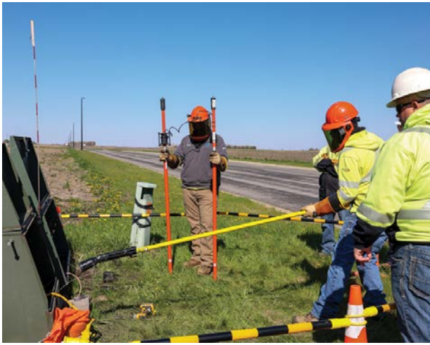
Most training takes place in de-energized stations, but the grounding and phasing stick activity gave participants exposure to energized grounding procedures. They learned how to ground lines and equipment and how to use phasing sticks when grounding and phasing cables.
