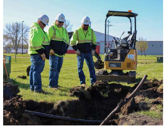
Participants learned cable design fundamentals, manufacturing basics, and proper preparation for termination. The session also covered reel handling and inspection, installation best practices, and common causes of cable failure.
