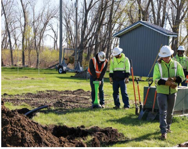
Participants at the 2026 Underground School track a directional drill's path at MMUA's Marshall training center. The school drew 54 utility professionals from Minnesota, North Dakota, and South Dakota.
