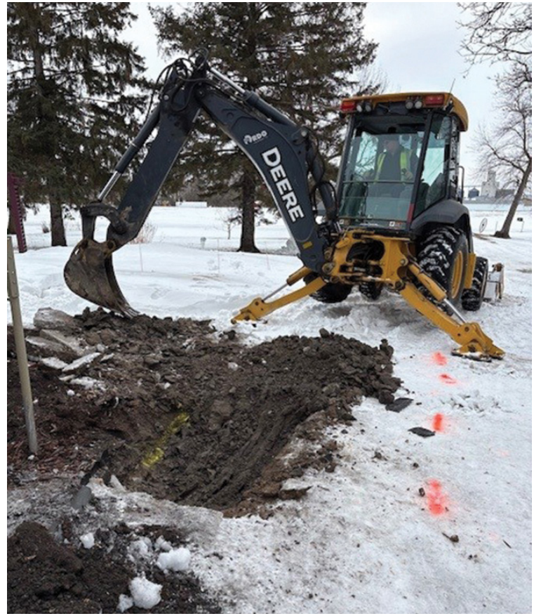
On site, Danielson operates a backhoe to locate the leaking gas line after emergency locate services were complete. Use of the backhoe was necessary because the frost depth was 3.5 feet, and standard bar holing tools could not penetrate the ground.
