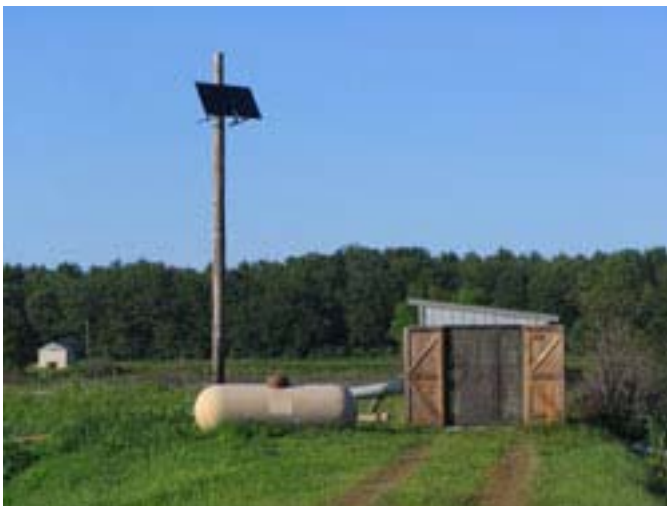
Solar Panel at Pump House
