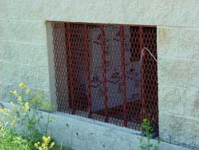
Metal Screen for Window Airflow/Vandals
