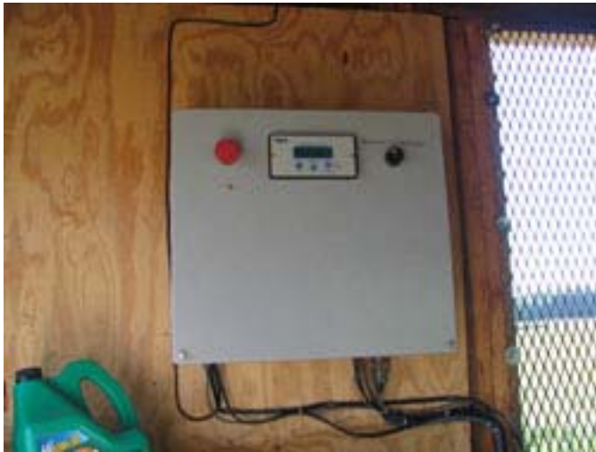
Controller in Pump House
