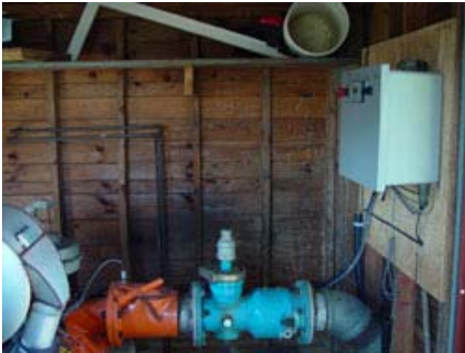
Control Box and Pump
