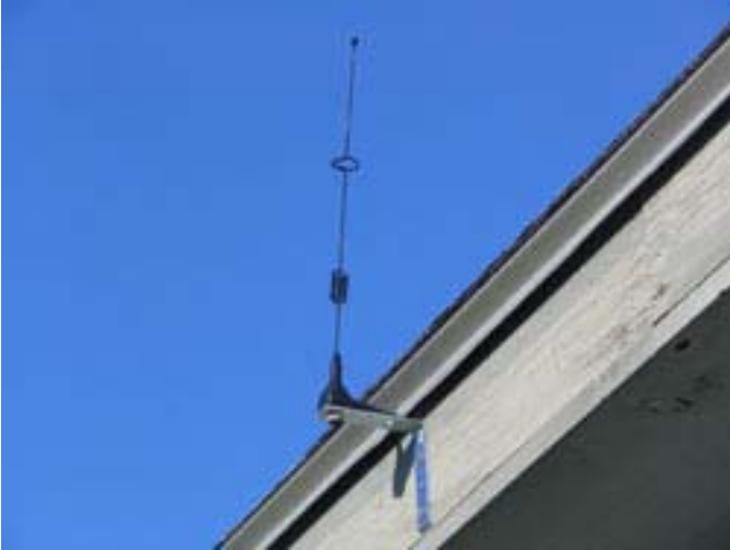
Antenna Mounted on Pump House Roof
