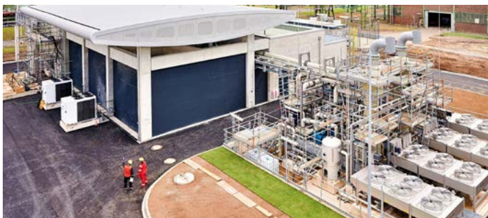
Europe's largest PEM hydrogen electrolyser, began operations at Shell's Energy and Chemicals Park Rheinland, producing green hydrogen. Photo courtesy of Shell
