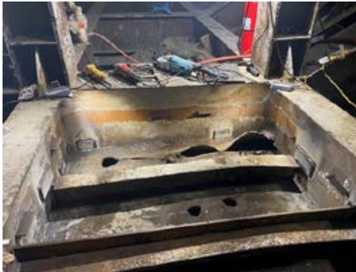
Figure 1: Damage with relief cuts
