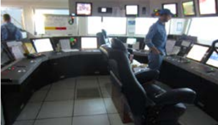
A fully digital bridge, linked to digital control and safety critical systems, and remote access.
