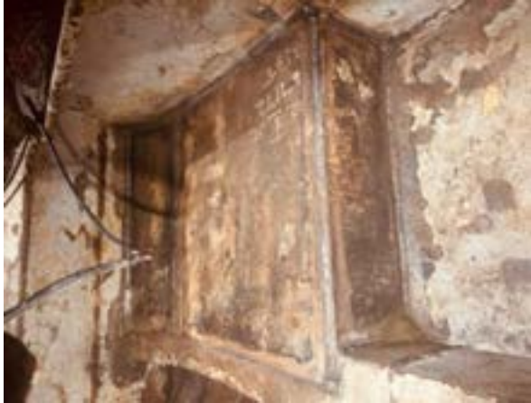
Figure 3: Forward internal cofferdam built around damaged area
