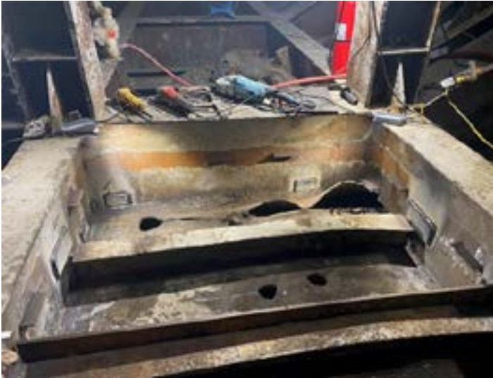
Figure 1: Damage with relief cuts
