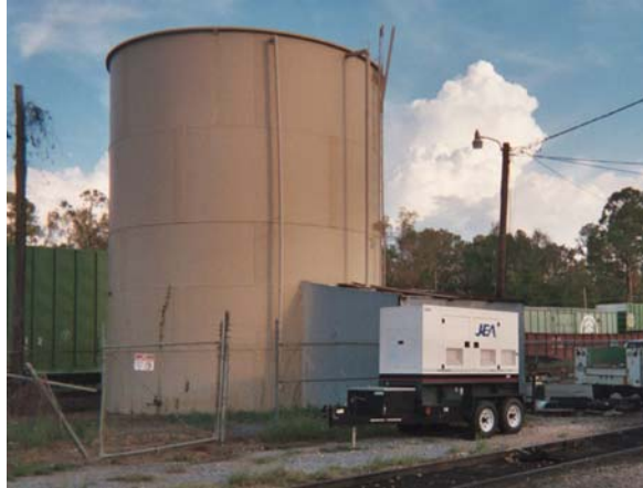
Large Commercial Generator Used to Power City of Kirbyville Texas Repump Station In aftermath of Hurricane Rita
