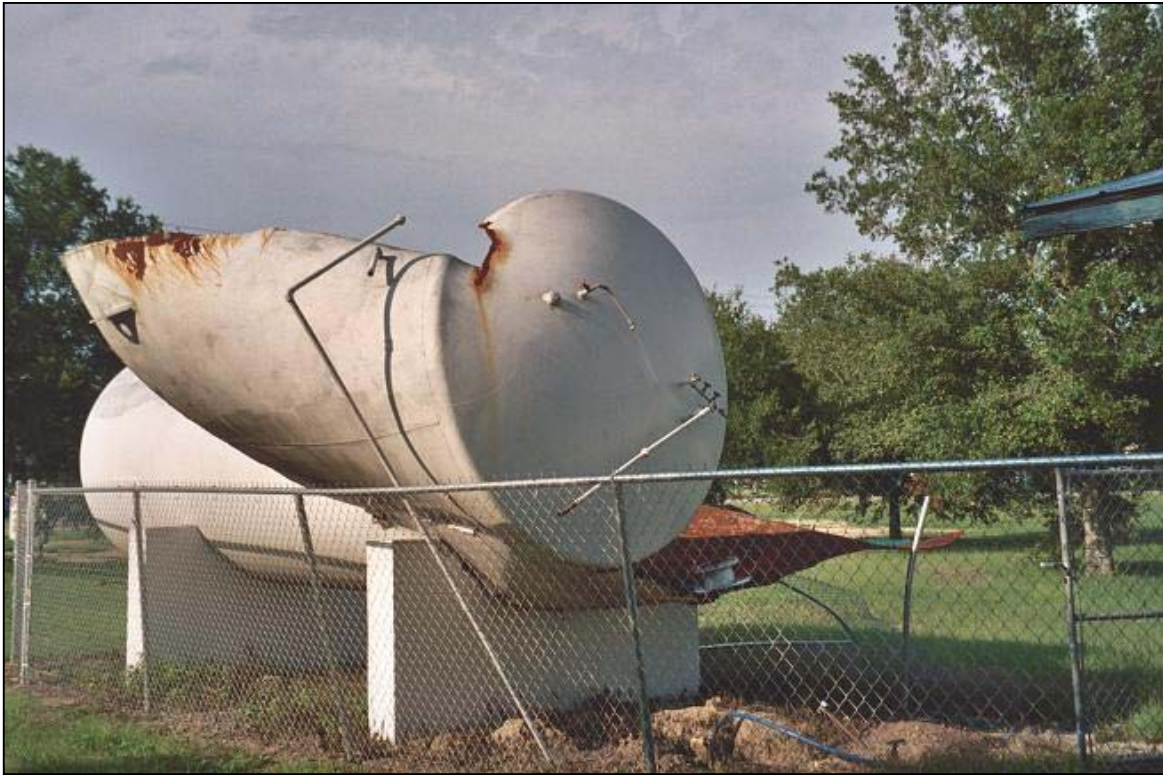
Hydropneumatic Tank Rupture
