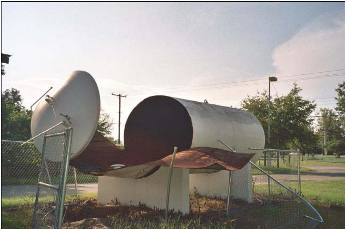
Hydropneumatic Tank Rupture
