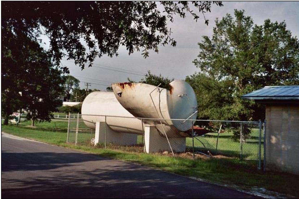
Hydropneumatic Tank Rupture
