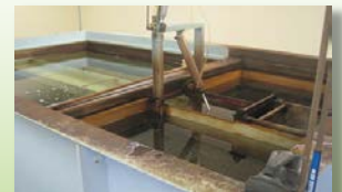
Drinking Water Treatment Plant
