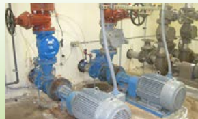
Booster Stations and Other Pumps
