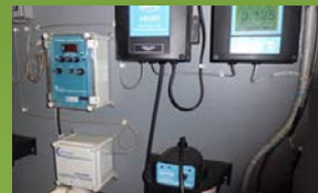
Instrumentation and Electrical Controls
