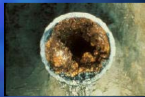
Heavily Tuberculated Water Main where pigging must be used to remove deposits
