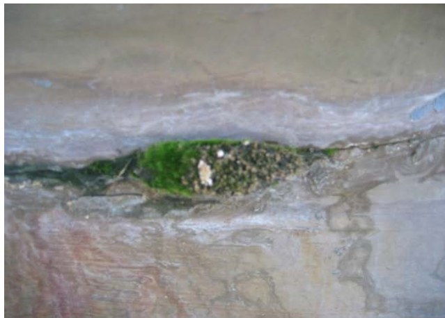
Cracks on a fiberglass tank
