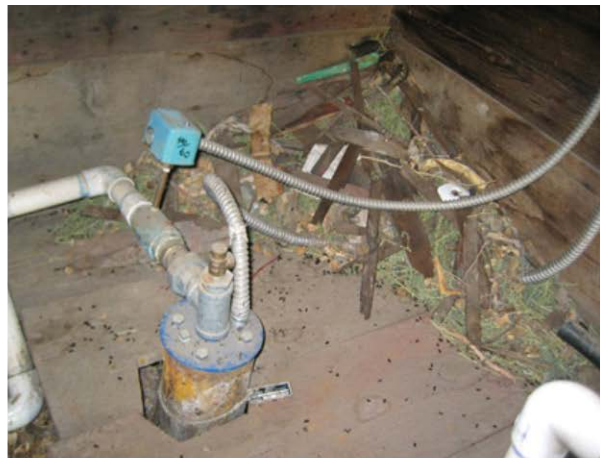
Rat droppings around the wellhead
