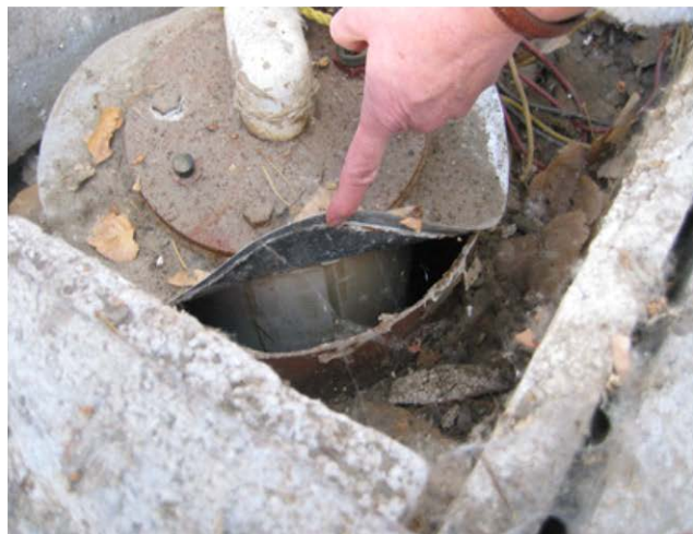
Seal on wellhead not watertight
