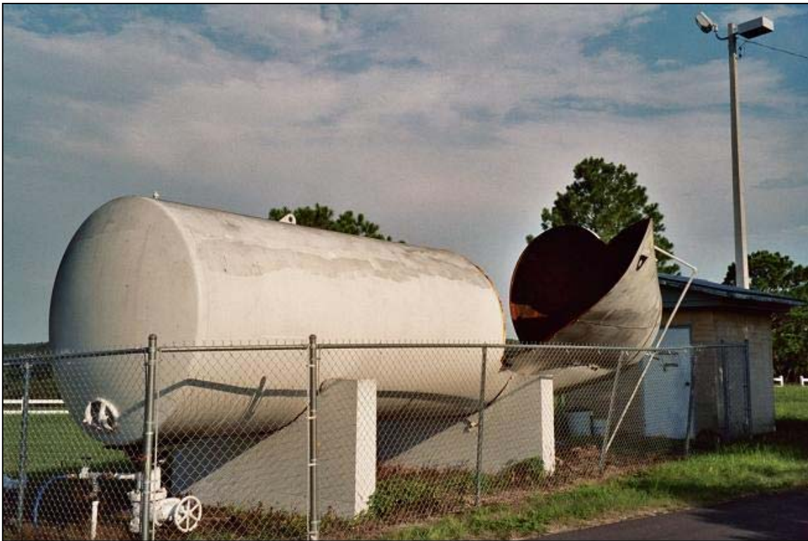
Hydropneumatic Tank Rupture
