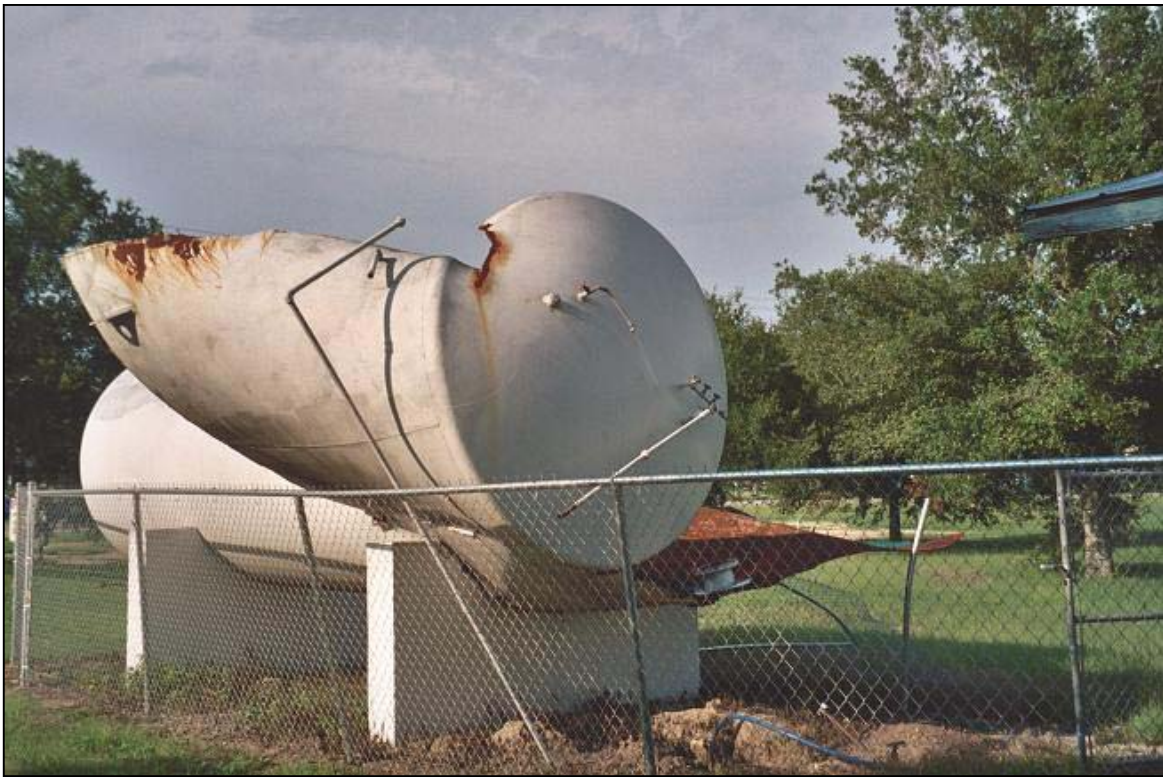
Hydropneumatic Tank Rupture
