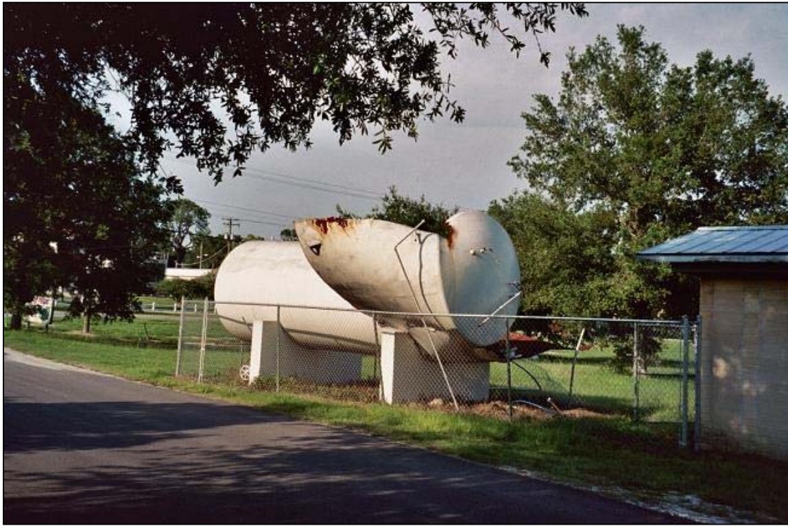
Hydropneumatic Tank Rupture
