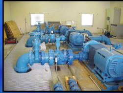
High Service Pumps
