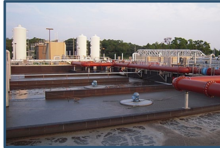
Wastewater collection and treatment
