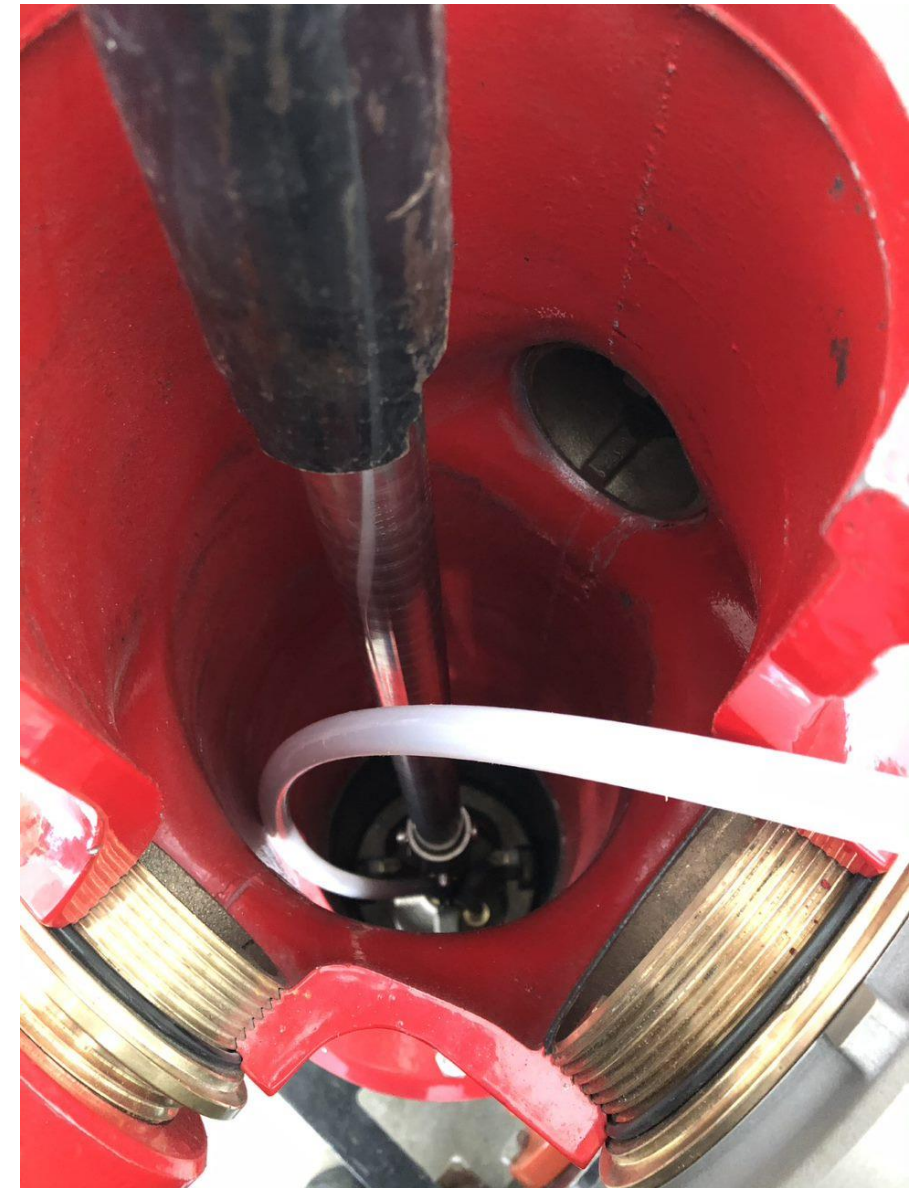
Internal Wiring & Cables
