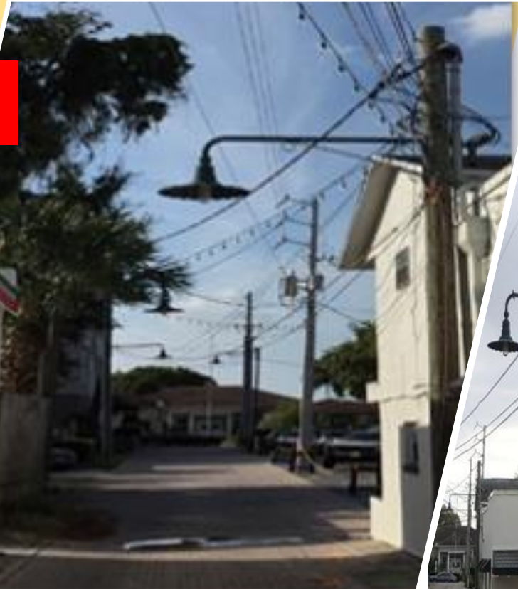
Large Secondary Cables
