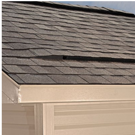
On roof intake ventilation
