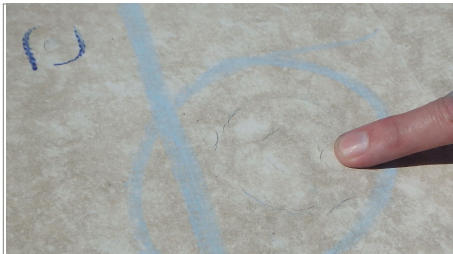
Star fractures on the backside
