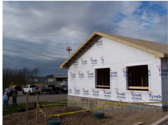
The fall took place from this structure. Photograph property of KY FACE Program
