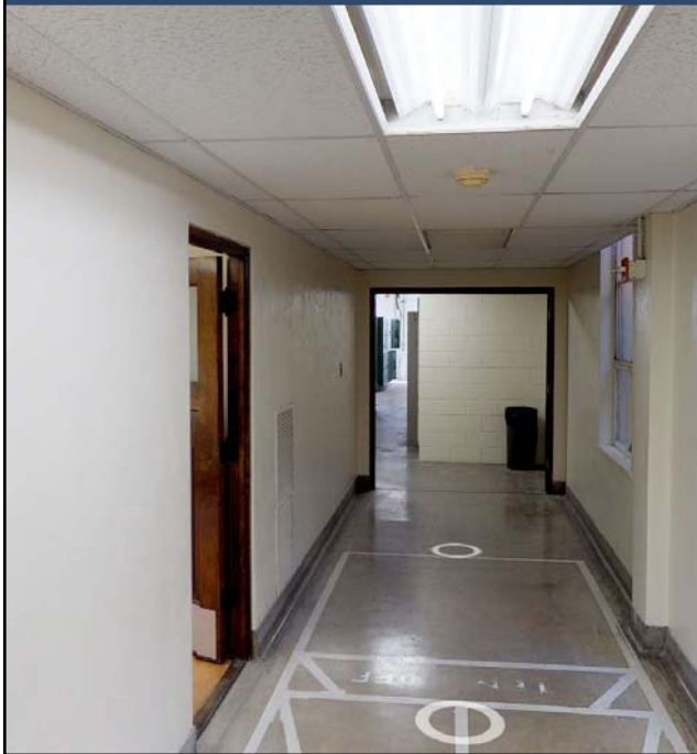
THE UNIVERSITY OF TEXAS AT AUSTIN | ANNA HISS GYMNASIUM | LEVEL 1 BEFORE AND AFTER
