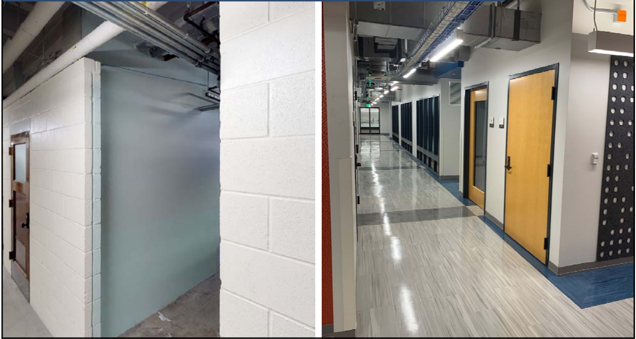
THE UNIVERSITY OF TEXAS AT AUSTIN | ANNA HISS GYMNASIUM | LEVEL 1 BEFORE AND AFTER
