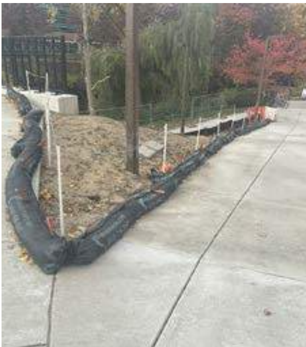
Erosion eels near pedestrian bridge
