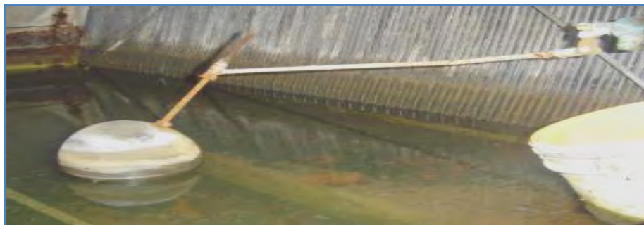
Figure 7.51 - Cooling Tower Float Valve and Overflow Pipe
