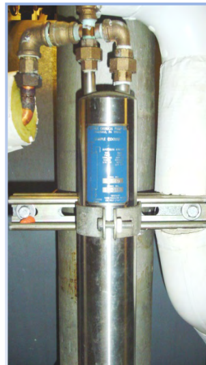
Figure 7.57 - Boiler Water Sampler Device
