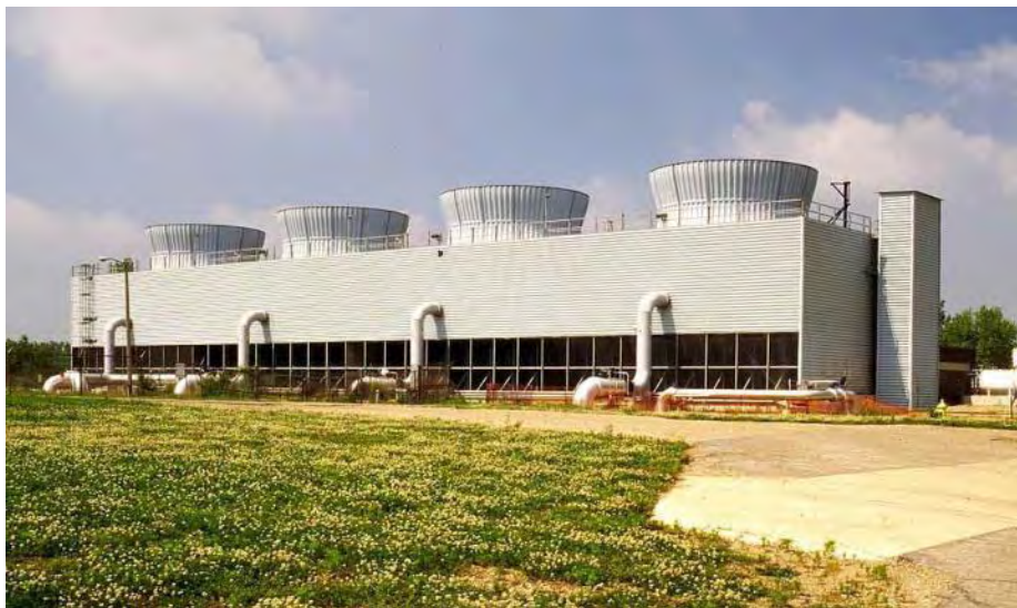
Figure 7.50 - Marley Counter-Flow Towers
