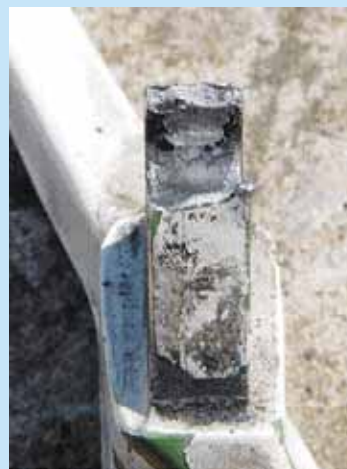
Figure 7: View of Failed Part
