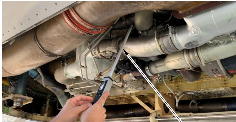
AIR CONDITIONING CHECK (EXAMPLE)
