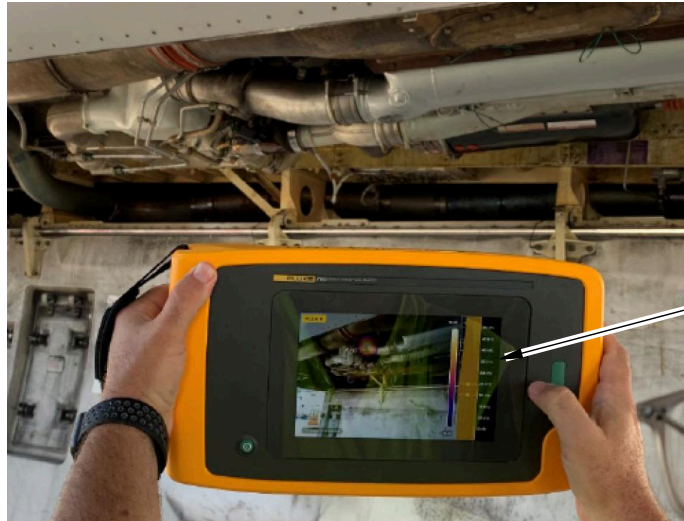
AIR CONDITIONING CHECK (EXAMPLE)
