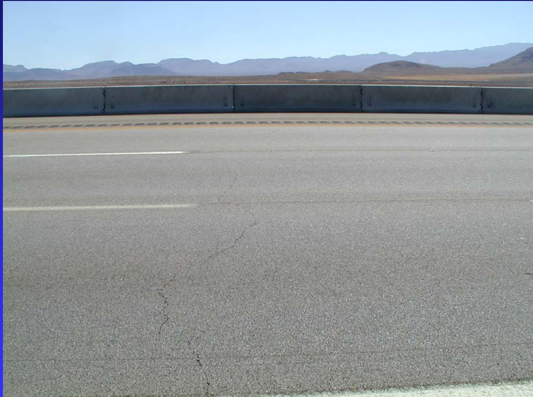
I-15 Reflective Cracking - 2002
