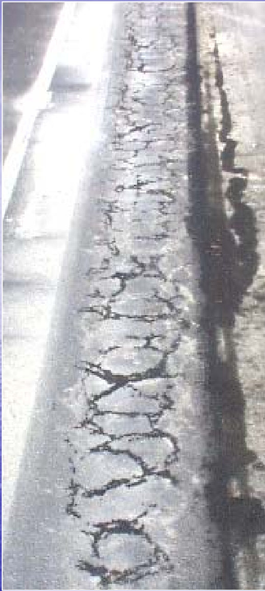
Lane 2 (Control) After 100,000 Loads
