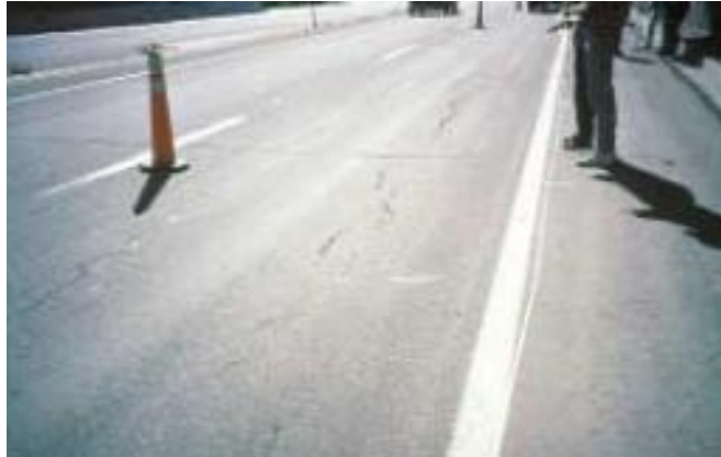
Low Severity Wheelpath
