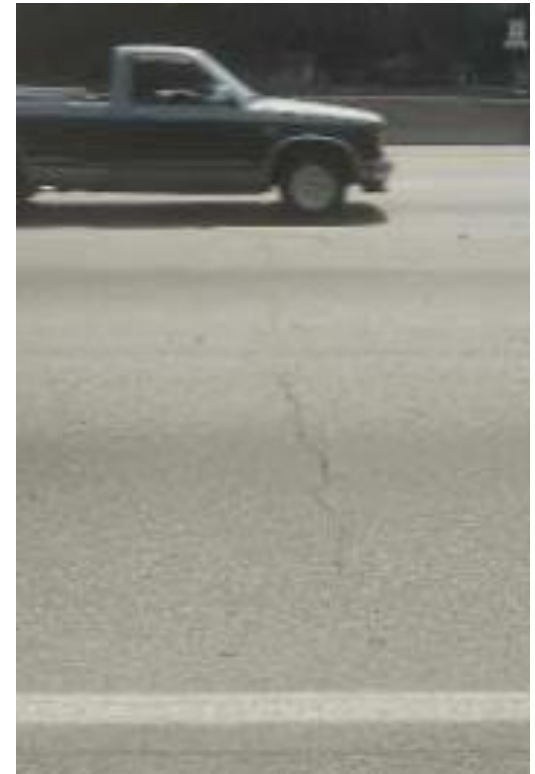
Low to Mod. Transverse Cracking
