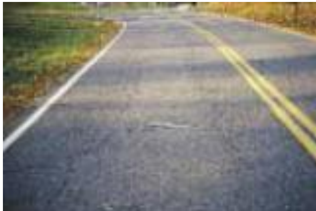
Low to Mod. Longitudinal Cracking
