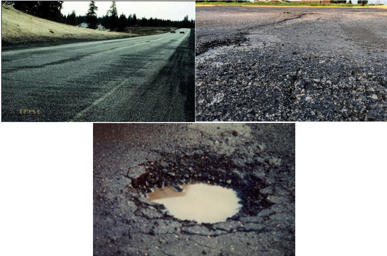
Figure 1. (Top-left) Stripping (Halim and Ramani, 2016), (top-right) raveling (RoadBotics.com), and (bottom) potholes (Williams and Breakah, 2010) in asphalt pavements
