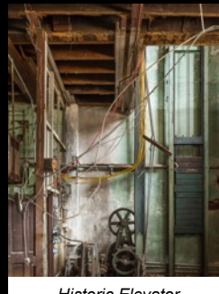
Historic Elevator Hoisting Equipment (2016)
