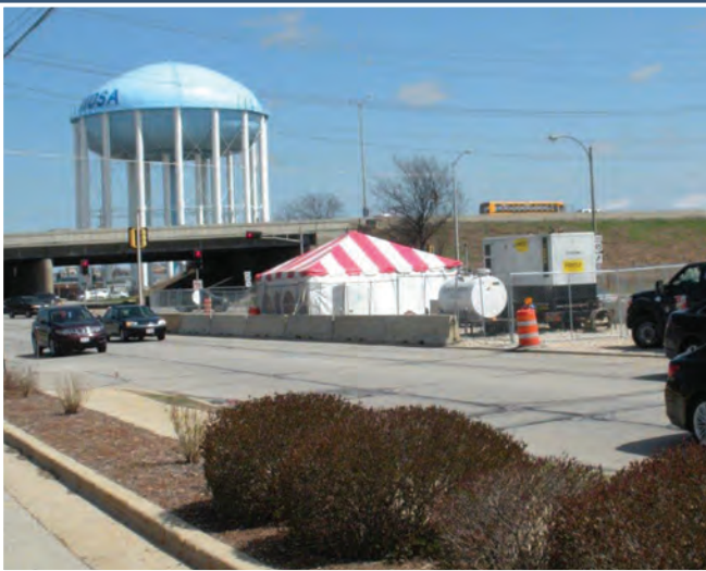
Wisconsin Ave. Transmission Main & Temporary Booster Station (in partnership with the City of Wauwatosa Water Utility)
