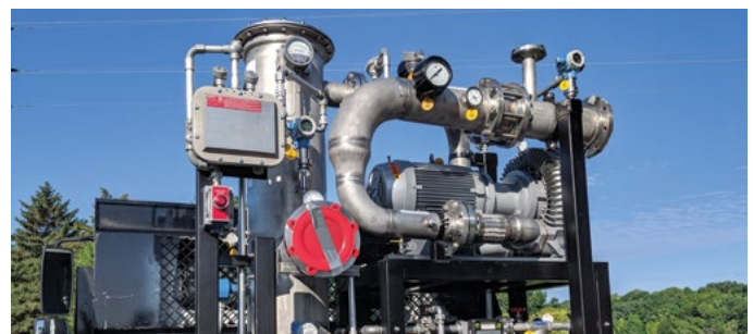
This compressor was a vital part of the stabilization and homogenization process for biogas.
