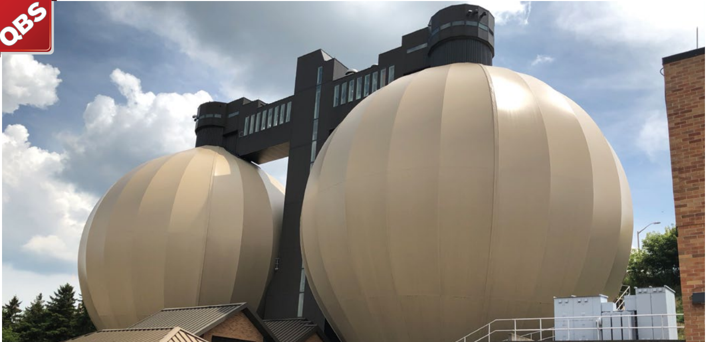
Two huge anaerobic digesters process billions of gallons of wastewater yearly.
