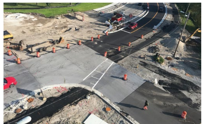
With smart construction staging, the road stayed open, preserving access to the medical complex.
