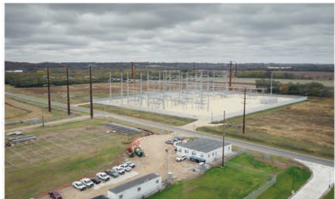
A new substation will improve energy transfer to the nearby City of Beloit.
