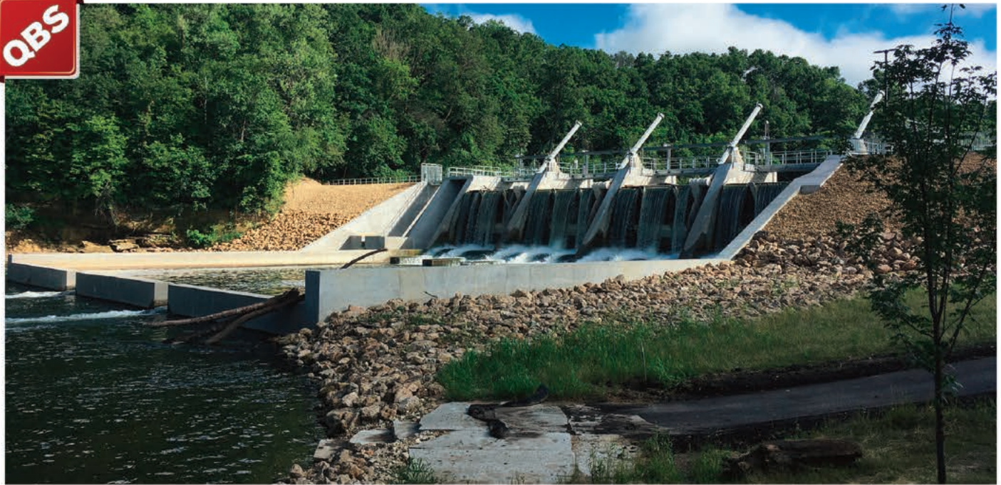
The new control gates allow proper water flow in addition to regulating temperature and sediment discharge.
