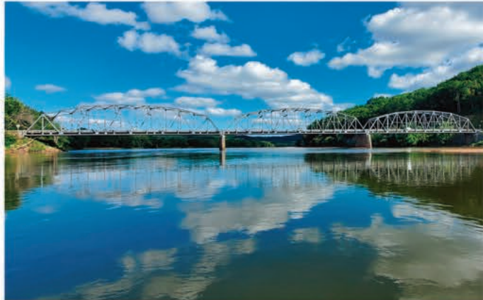
The rehabbed structures ensure safety for the over 2,000 cars that travel across the Wisconsin River daily.
