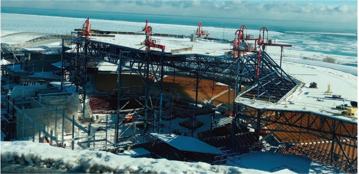
A 300-ton center portion of the roof was lifted in the middle of winter to stay on schedule.
