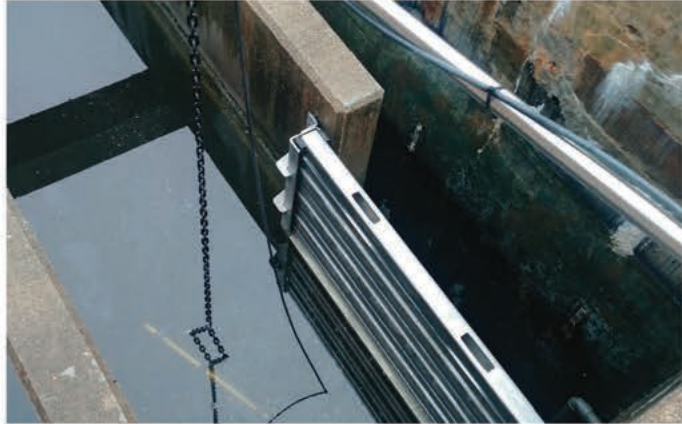
Sensors in the water provide information to a control center that adjusts the strength of the UV lights to meet needs.
