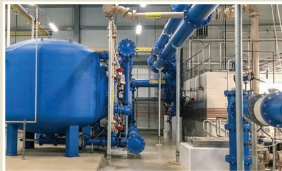
Elkhorn Water Treatment Plant
