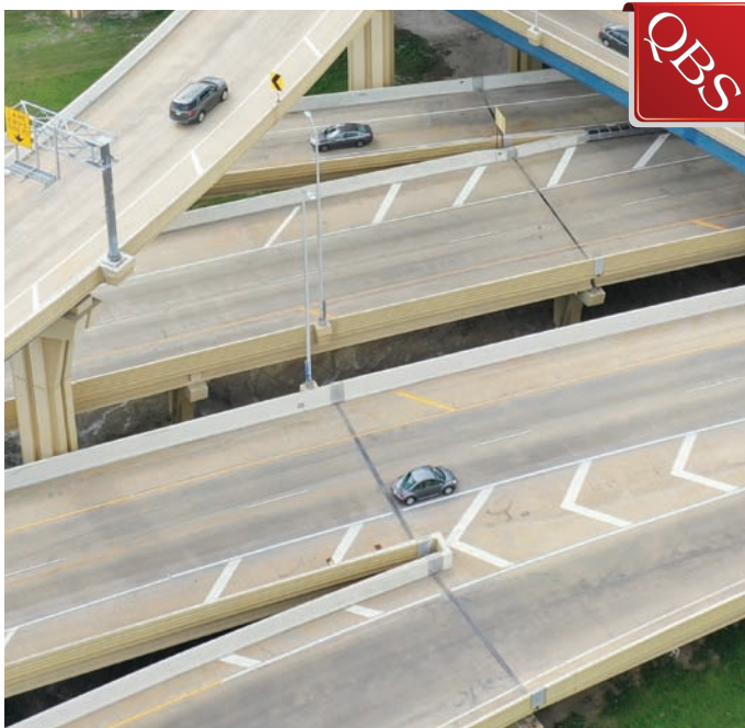
The PPC overlay preserves the steel reinforcements in the concrete, preventing corrosion and extending the overall life of the project.
