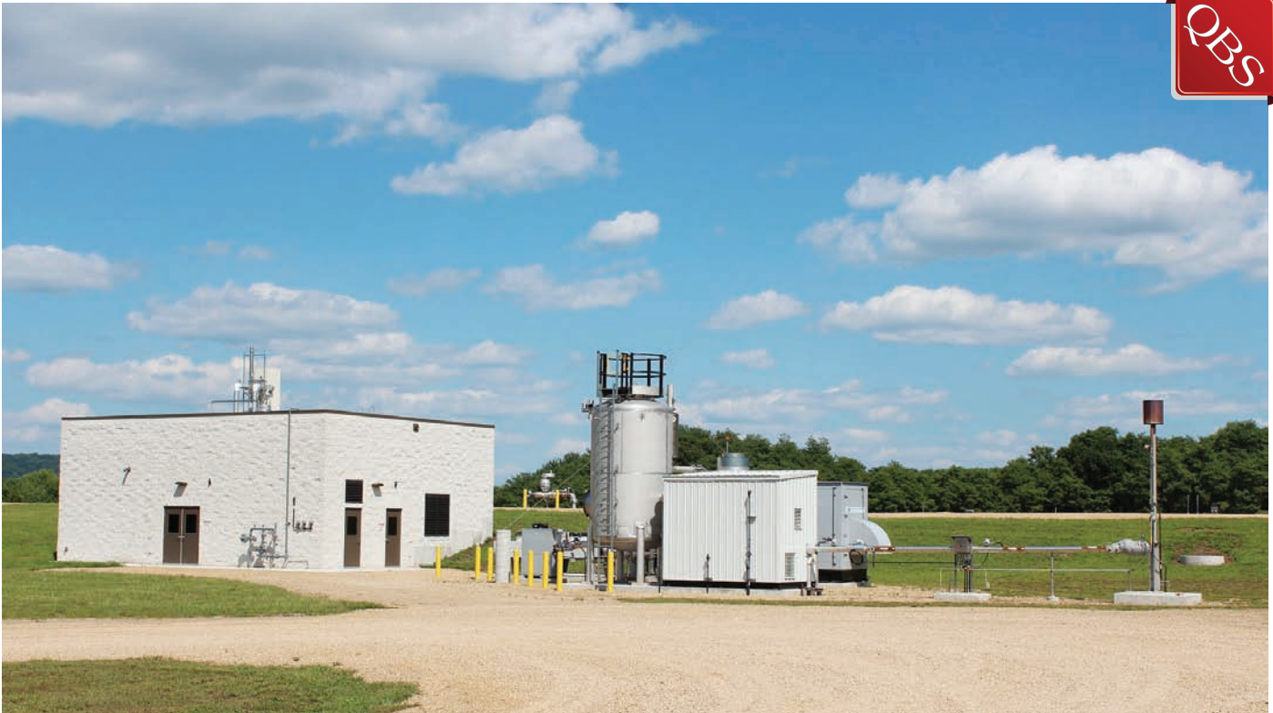
TOP: With a small footprint, the new plant delivers large results by dealing with all of the waste generated by the cheese company. BOTTOM: The new anaerobic lagoons produce biogas that is immediately funneled into a generator for the facility.
