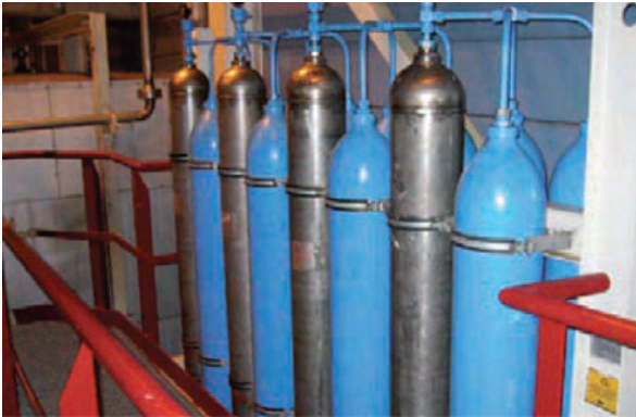
Figure 60: Storage rack with bolted cylinder brackets
