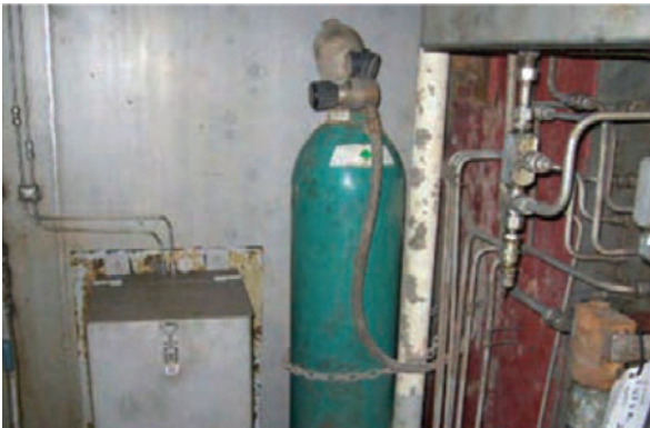
Figure 61: Temporary storage of cylinders secured with chain
