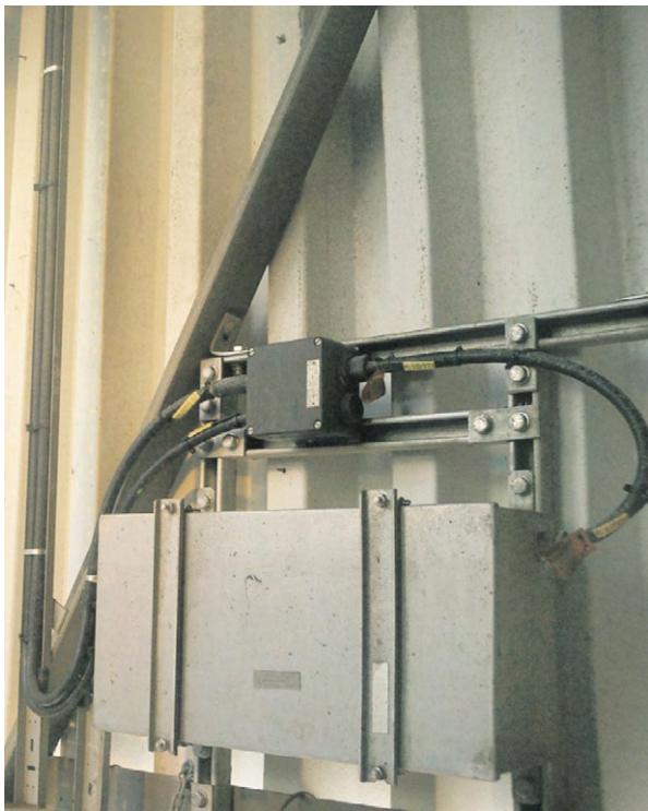
Figure 46: Junction box and cabinet
