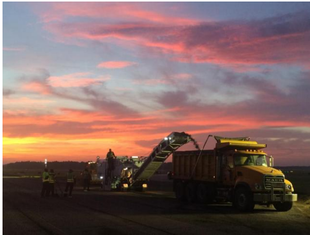
V.E. Whitehurst & Sons, Inc. for their project on Runway 7/25 at the Gainesville Regional Airport in Alachua County. Tonnage: 11200
